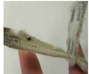
Frayed and worn connecting point.
