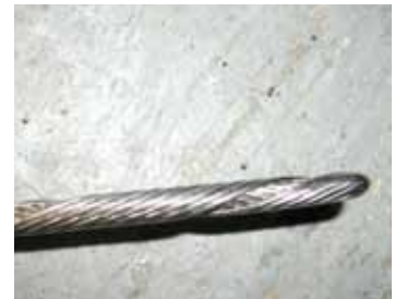
Non-approved metal cable and metal unraveling.
